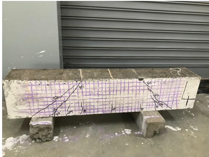
Fig 13: Crack pattern developed in a beam
